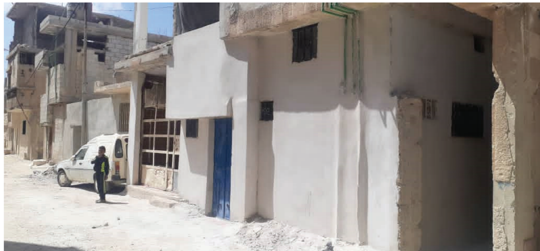
Self-help minor shelter repair conducted by a pilot project with UN Habitat in Dera'a camp. © 2022 UNRWA Photo
